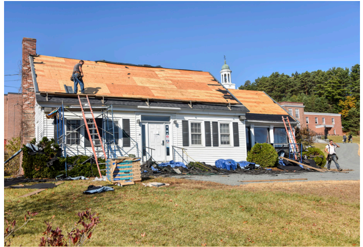
Workers are pictured here removing the last of the deteriorated shingles on Thompson Cottage. While this project has been completed, the John L. Norris, Jr. Center for the Arts will be the next building to have its roofing replaced.
